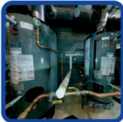
Mechanical Controls Upgrades
