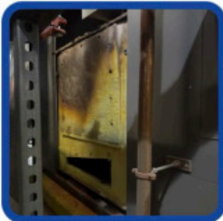
Fire Damaged Boiler
