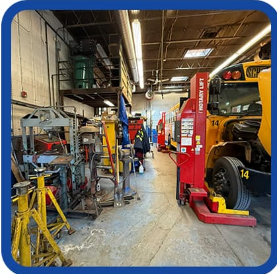
Unsafe Clearance for Personnel, Equipment & Buses
