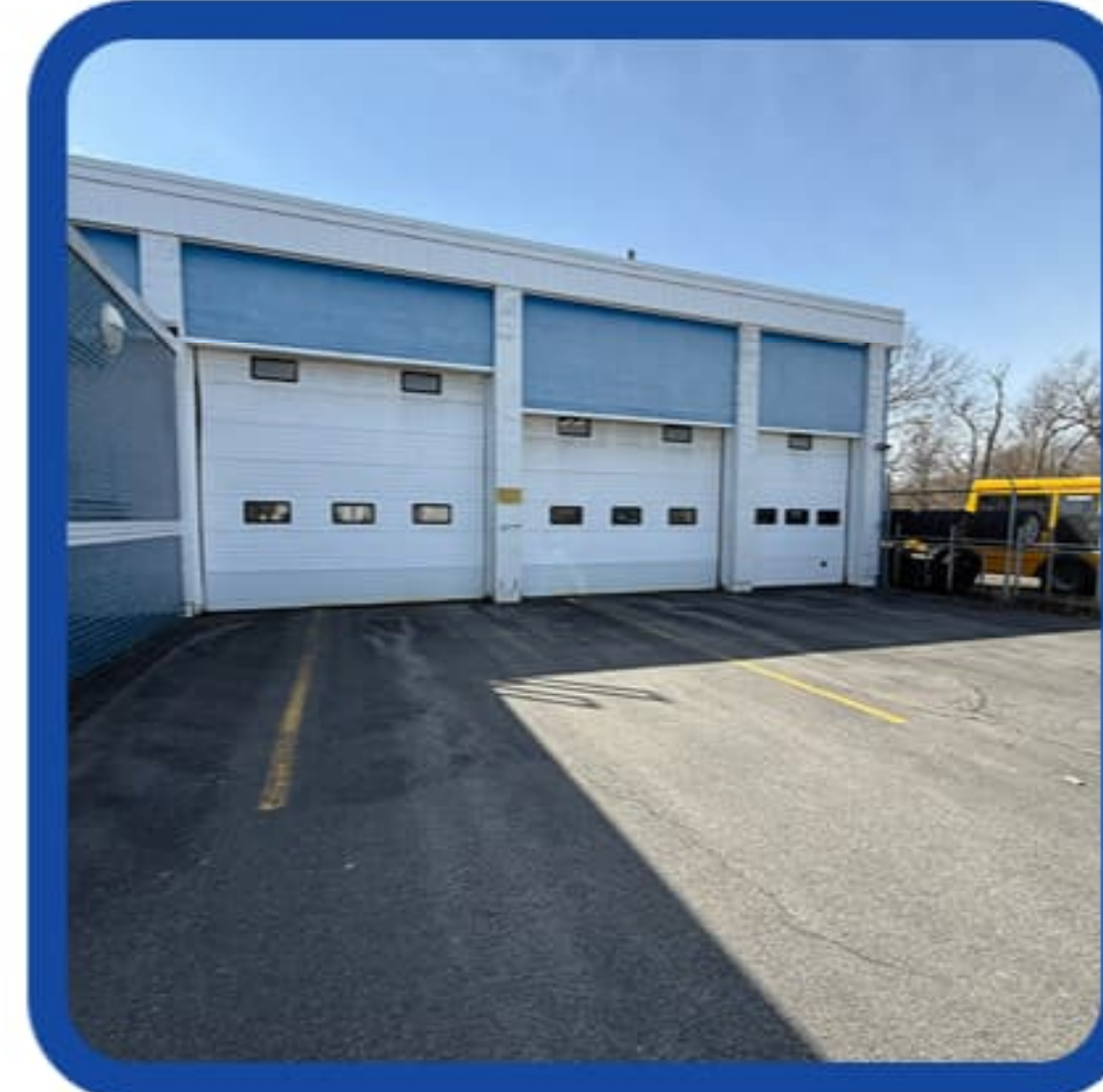
Undersized & Unsafe Overhead Doors
