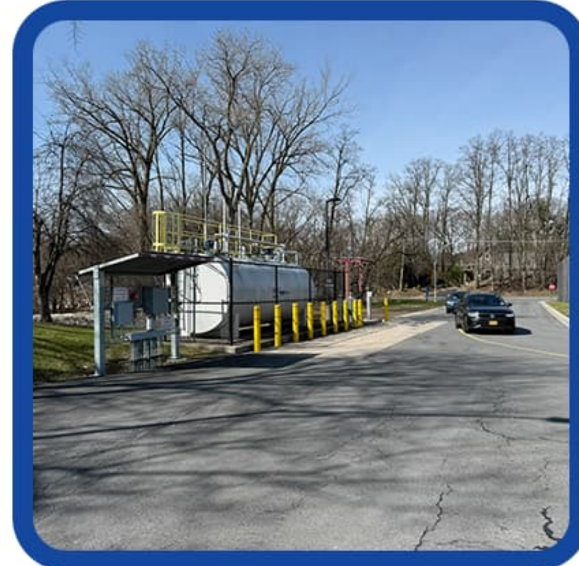
Unsafe Fuel Tank Location in Drive Lane
