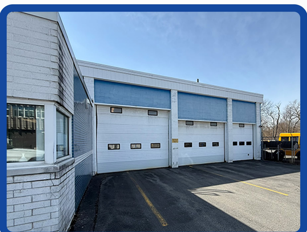
Undersized and Unsafe Overhead Doors
