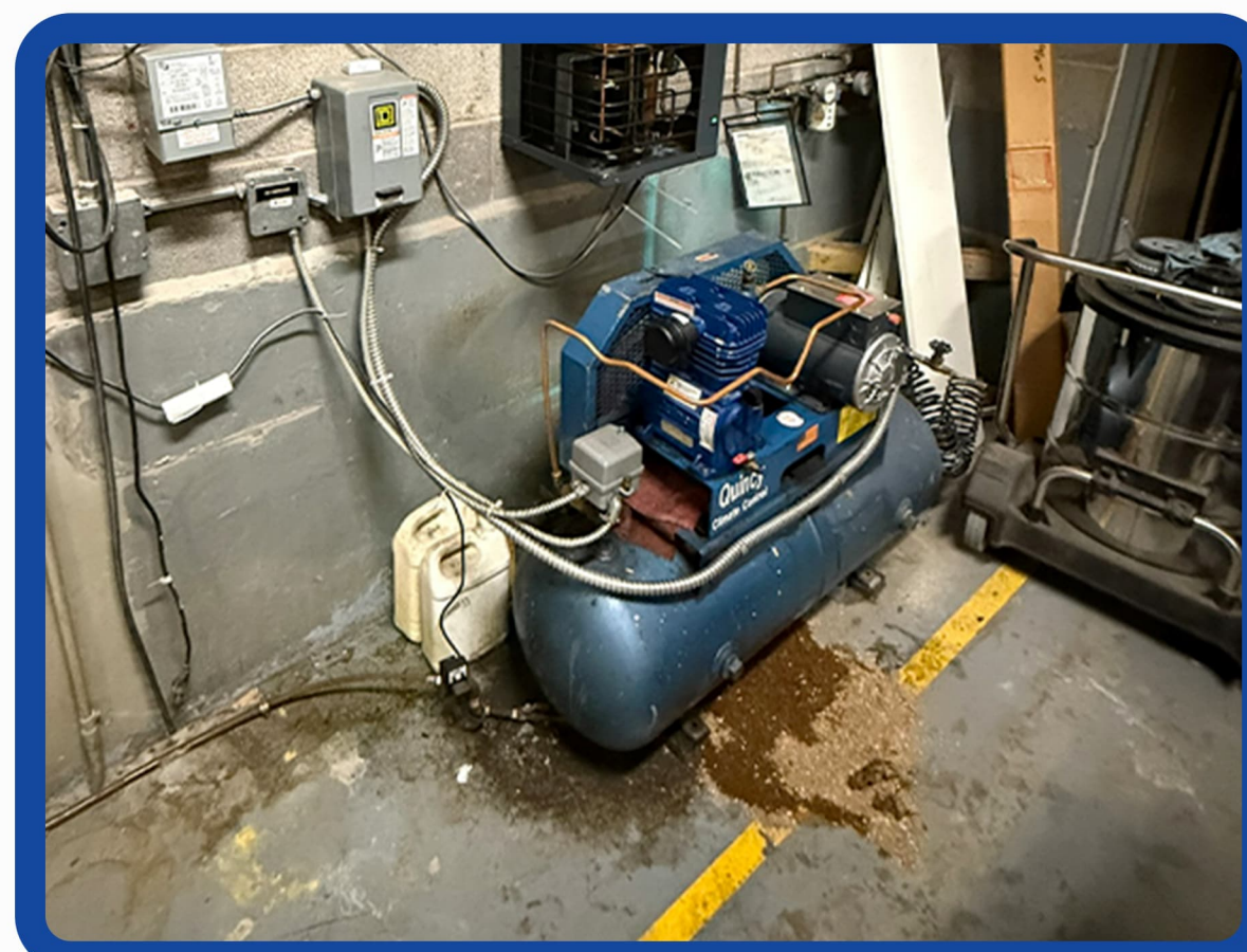
Outdated Mechanical Equipment
