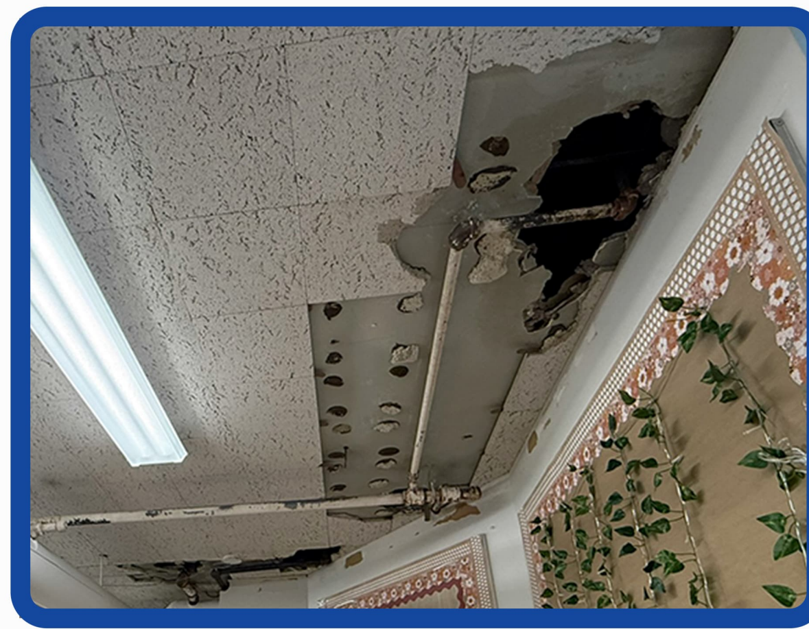
Replace Damaged & Out-Dated Ceilings
