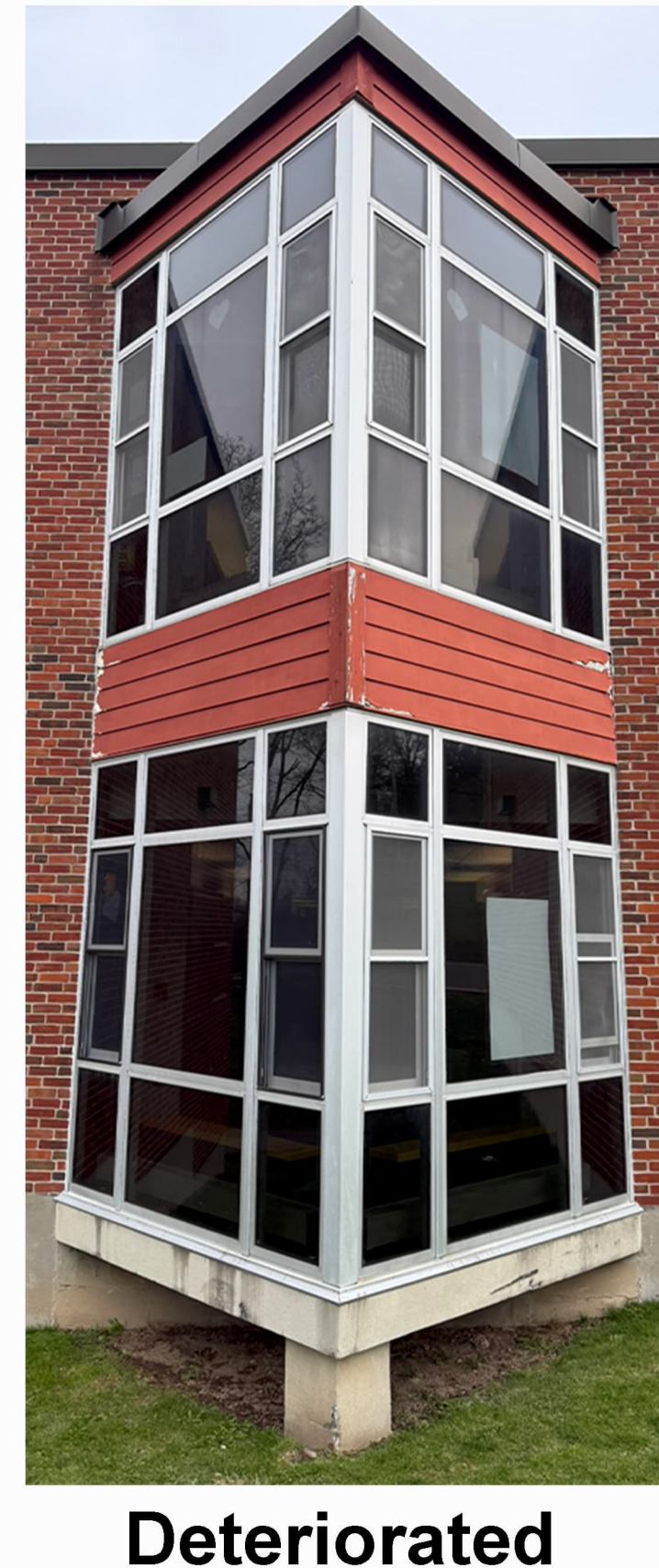
Deteriorated Exterior Siding
