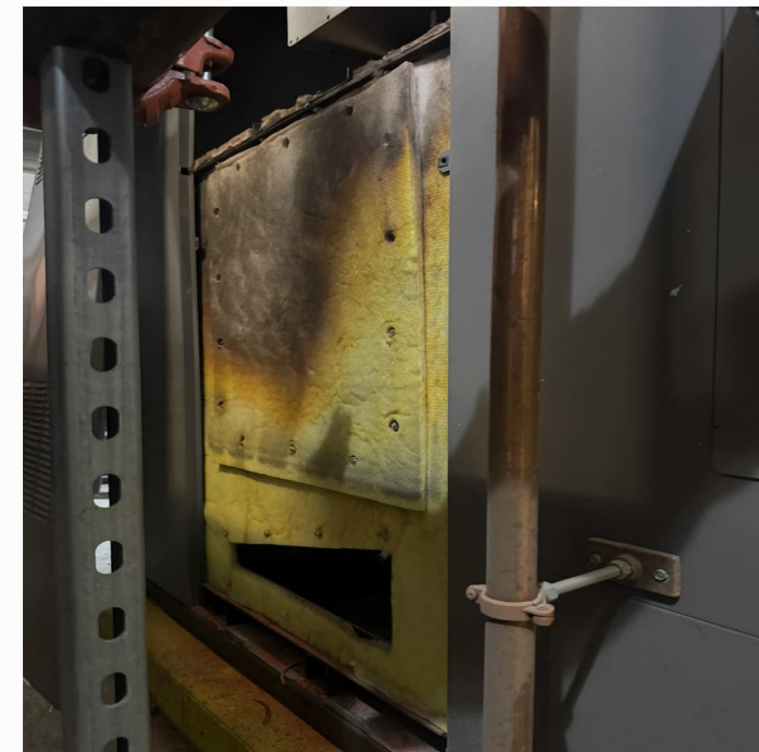
Fire Damaged Boiler
