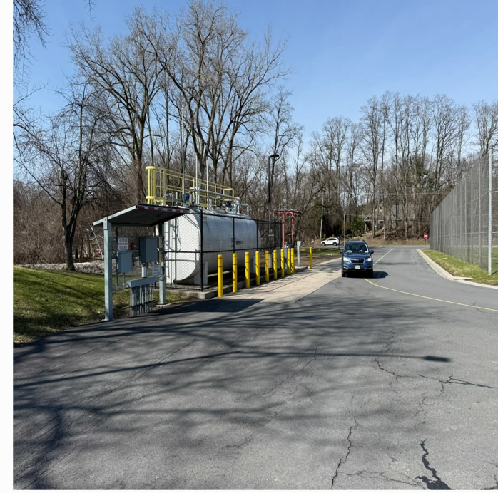
Unsafe Bus Fuel Station in Drive Lane
