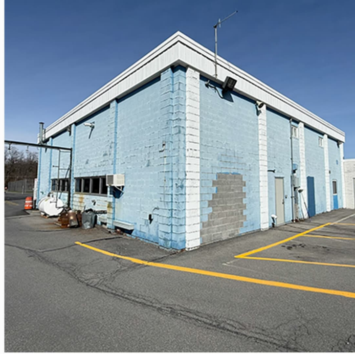
Bus Garage Struct. Wall Damage
